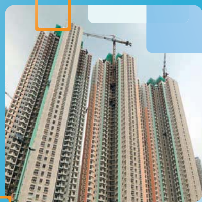
Redevelopment of Sau Mau Ping Estate Phase 14 秀茂坪邨第十四期重建項目工程
