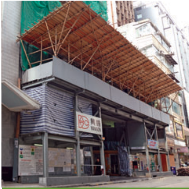
Construction of the proposed office/commercial development at 33 Cameron Road in Tsimshatsui 位於尖沙咀金馬倫道33號之建議辦公／商業發展項目
