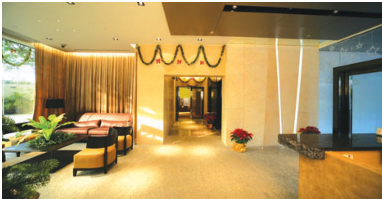
Renovation work for the lobby at Belgravia at 57 South Bay Road 南灣道57號Belgravia大堂之維修工程
