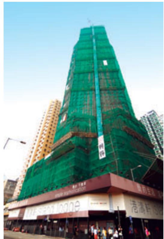
Construction of Island Lodge at 172-186 Java Road in North Point 興建位於北角渣華道172-186號之港濤軒
