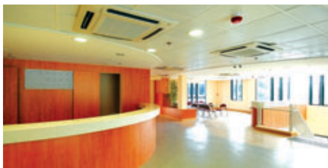
Supply and installation of false ceiling at Hong Kong Anti-Cancer Society Jockey Club Cancer Rehabilitation Centre at 30 Nam Long Shan Road in Wong Chuk Hang 為黃竹坑南朗山道30號香港防癌會癌症康復中心供應及安裝假天花
